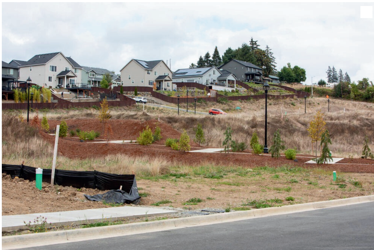
Workers continue to build houses in the subdivision Lockwood Meadows as families move into the newly completed homes. (Lizz Giordano/Cascade PBS)
